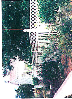
Landscaping shall be provided to adequately screen utility pedestals and transformers.
